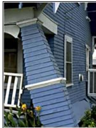
Figure 3-2 Earthquake Damaged Porch
