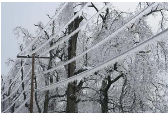
Figure 3-11 Ice Covered Power Lines
